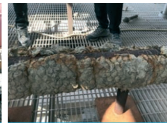
3) Corroded Section Under Insulation
